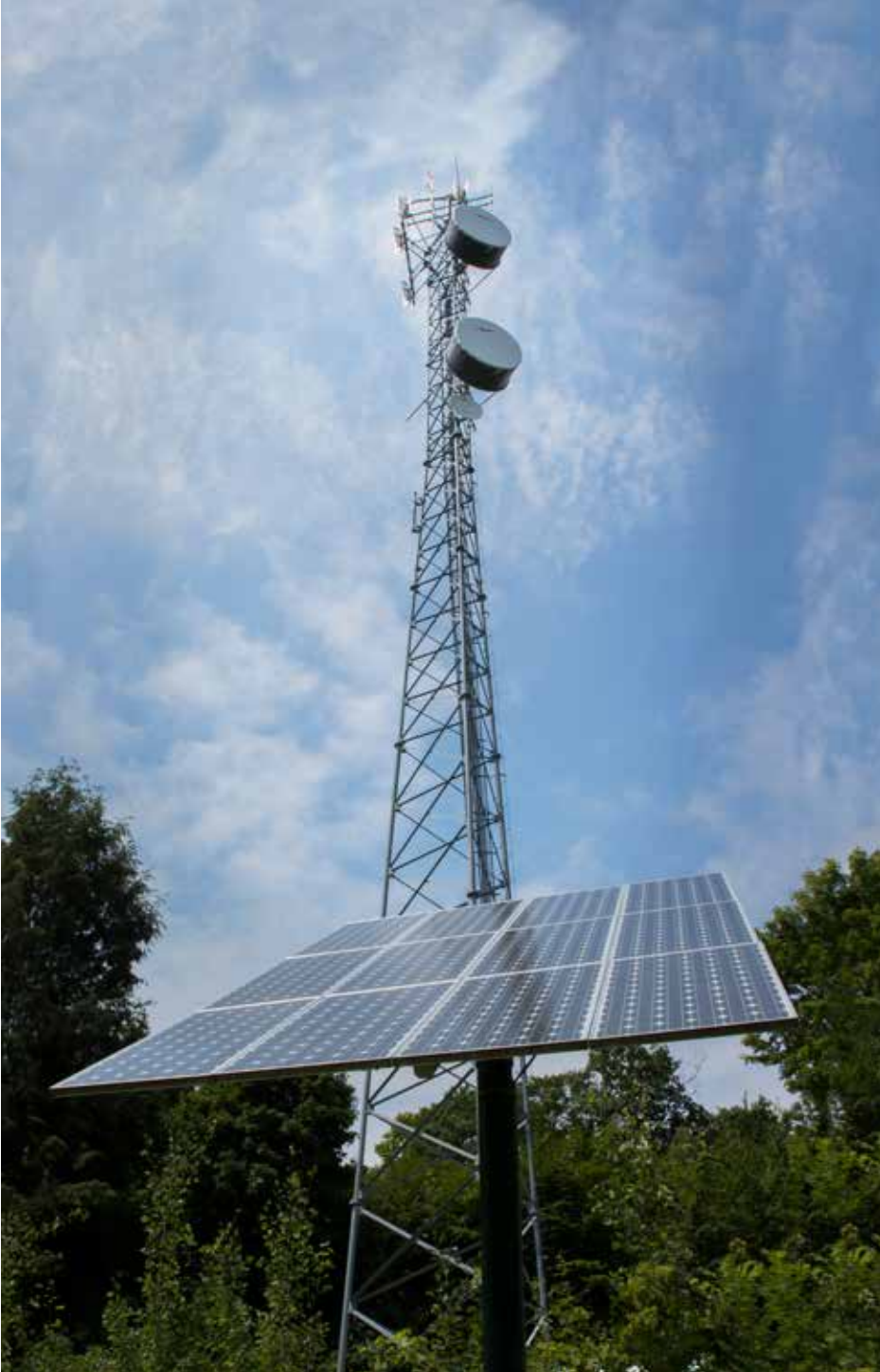
A Chambers Island cellular tower for Nsight
